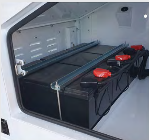
3 x 200ah LiFePO4 Batteries
