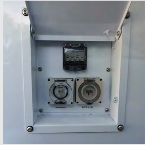
Inverter & 240V Charger
