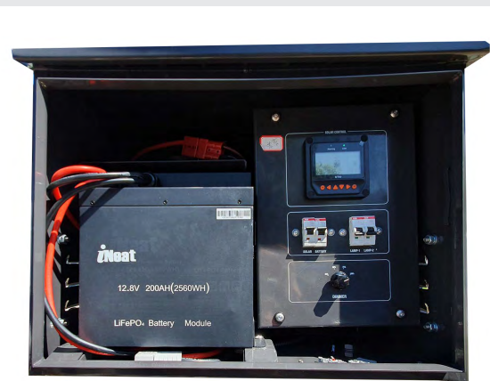
Battery and Control Box
