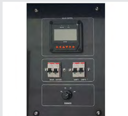
System Control Panel
